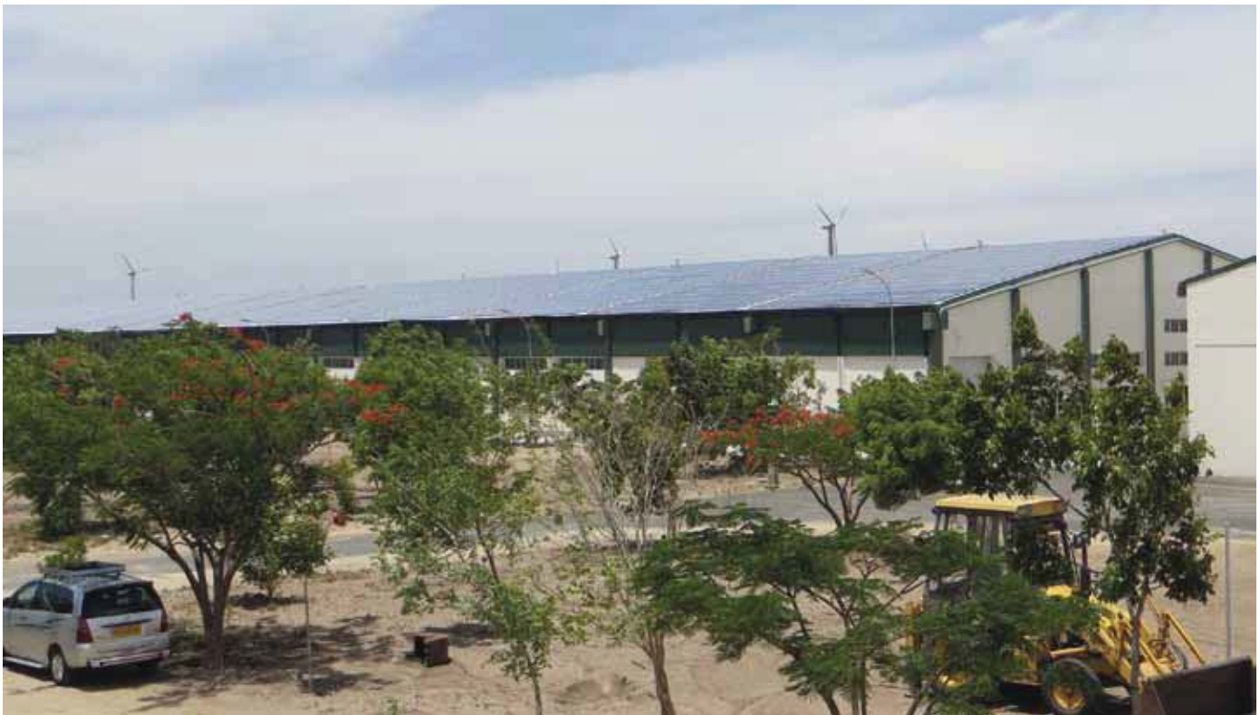
This diesel hybrid system in India is another example of the cost-savings in these fuel save control systems. SMA was also responsible for this installation.
