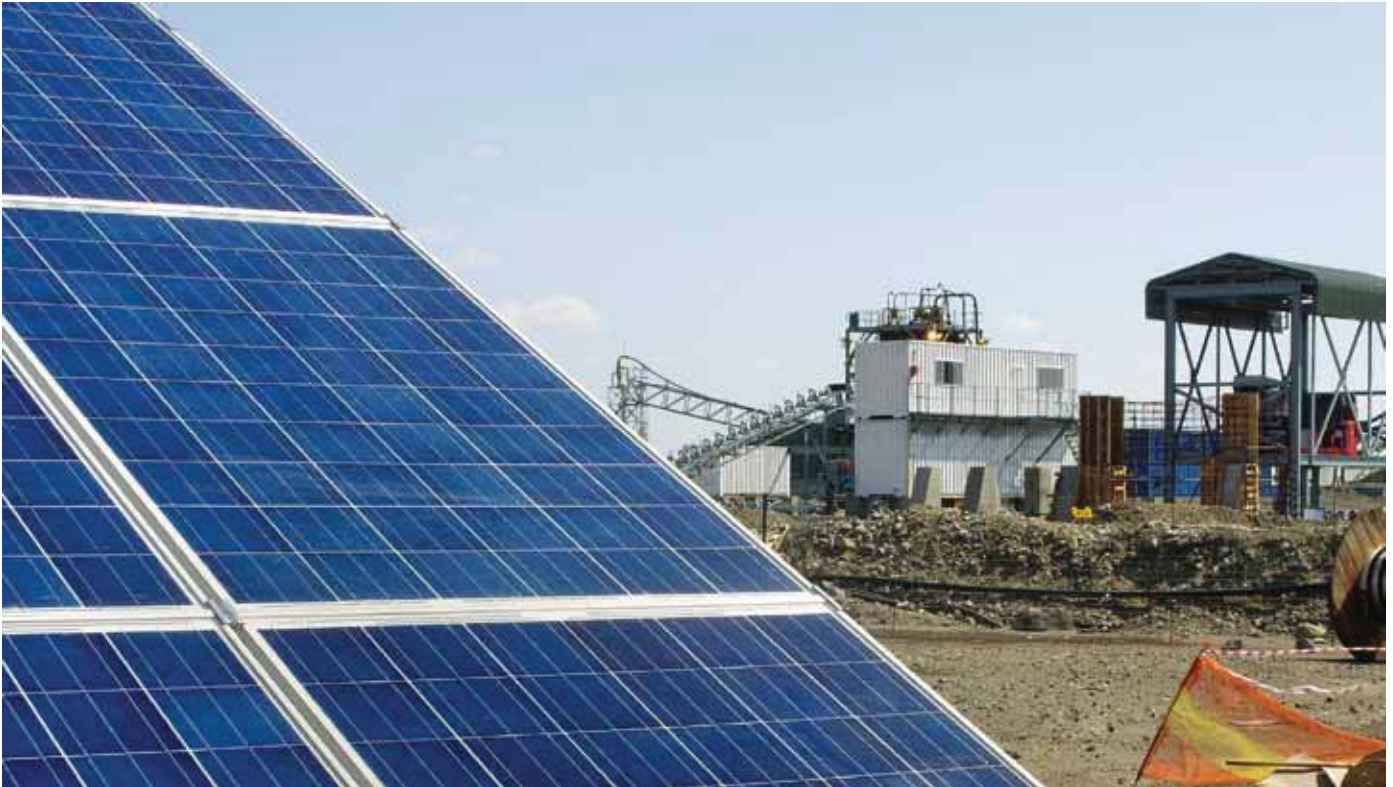
Photovoltaic systems can substantially reduce the operating costs of industrial plants – like the standalone power system, which SMA equipped with the required fuel save controller, in this mine in South Africa. Diesel generator output: 2 x 800 kVA; photovoltaic output: 1 MWp; savings according to SMA: up to 450,000 liters of diesel per year.
